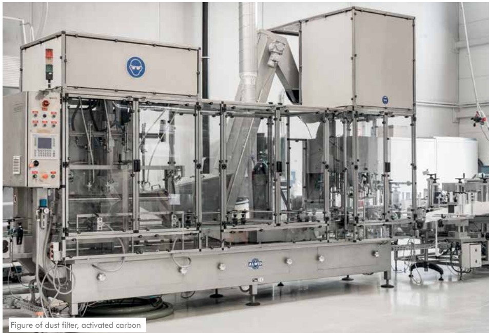
Figure of dust filter, activated carbon
